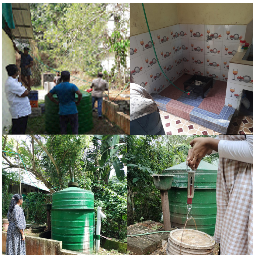
Installation of biogas plant at girls hostel and biogas is utilized for cooking purpose.
